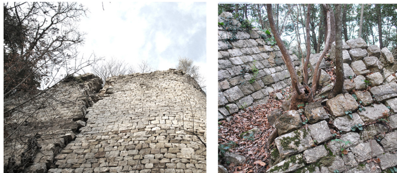
Fig 14. Main degenerative phenomena of the fortification.
